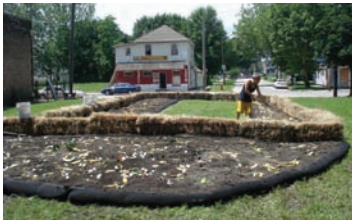
City Fresh worked with Filtrexx International to install a garden on a vacant lot in Cleveland. Straw bales were used to frame the garden (top). Cardboard was laid down first, and then compost-filled socks were placed on top (middle). Soil was added to fill in around the socks. Food scraps were scattered on top to be tilled into the soil (bottom).
